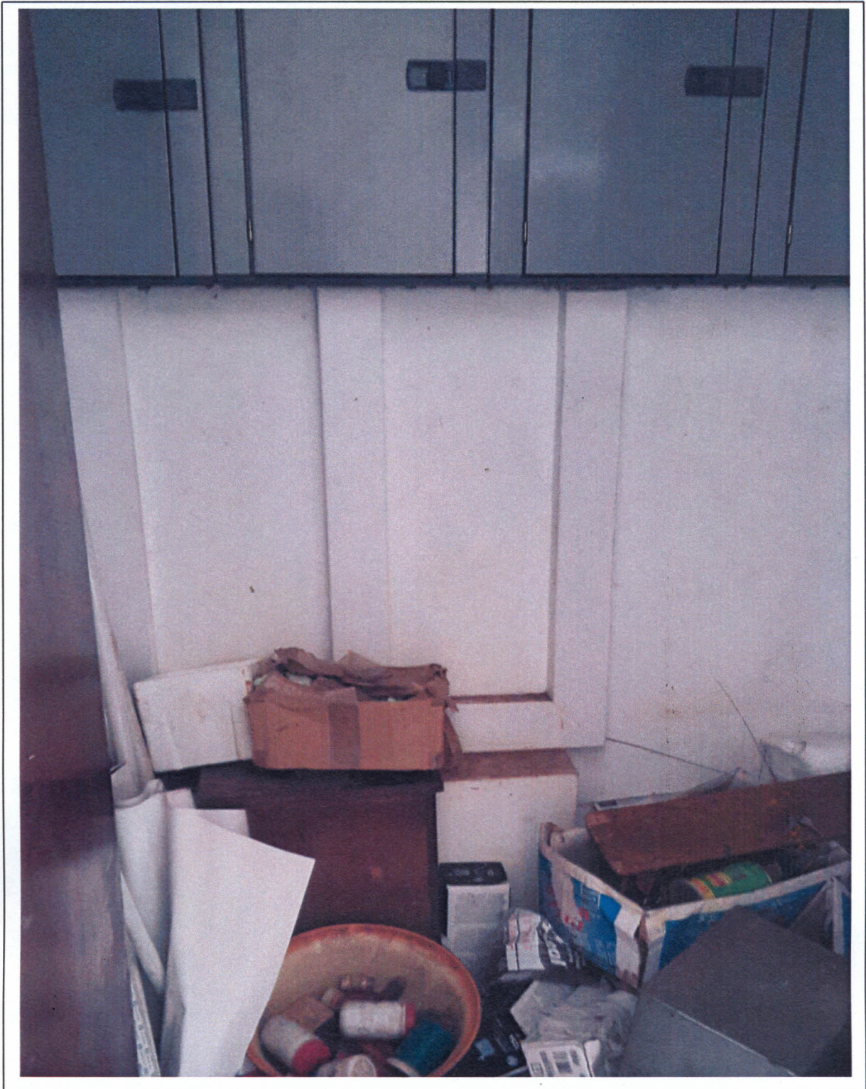
Fig. 7 . Electrical Switch Cupboards Being Used As Storage of Potentially Flammable Material
