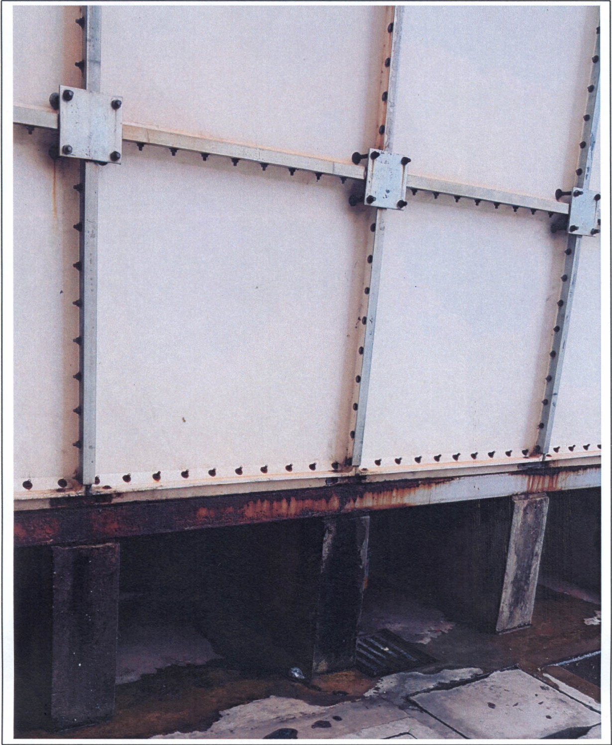
Fig. 2. Leaking Water Tank Behind the Main Building
