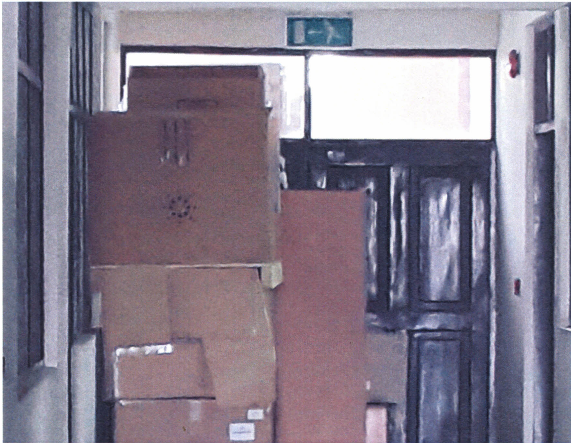
Fig. 8 A Picture Showing One Of The Fire Exits Blocked With Cardboard Boxes
