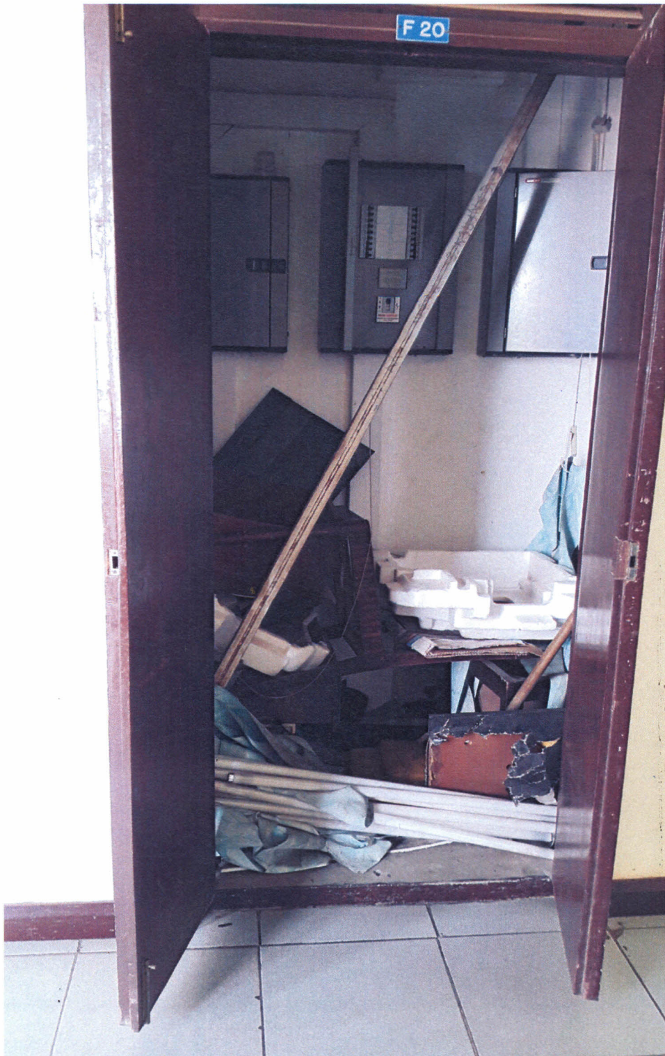
Fig. 8. Another Picture Showing Electrical Switch Cupboards Being Used As Storage of Potentially Flammable Material
