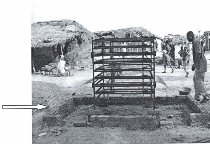
Fig. 23 Mounting and fixing of metal frame unto blocks; and positioning chicken mesh (arrowed) with mortar
