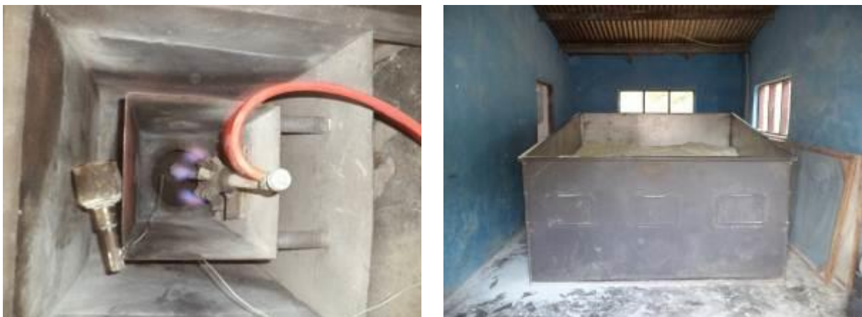
Figure 10. Gas burner and body of the bin dryer at Andyco Company Ltd., Kpevein the Volta
