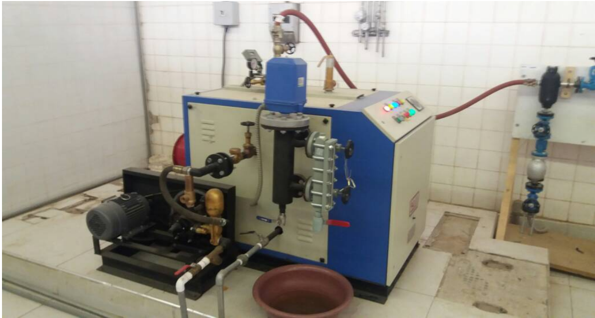
Figure 2: Electric steam boiler
